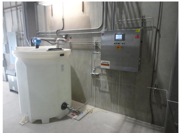
Figure 2 Indoor Urea Tank
