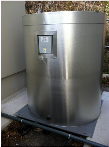
Figure 1 Outdoor Urea Tank Heated and Insulated
