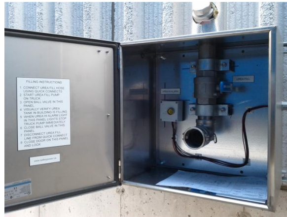
Figure 3 Urea Fill Station
